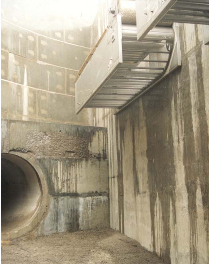
Inchcape (Station de pompage), UK ( 3,000 l/s)
