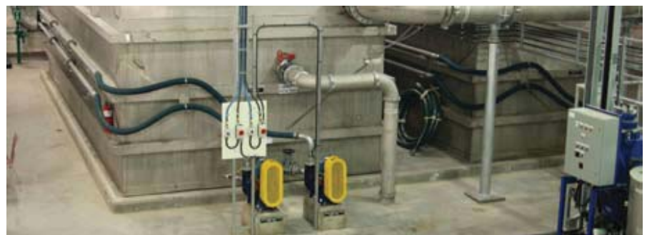
The Red Lake Mine's arsenic treatment plant includes two ACTIFLO® ACP-750 units with a total flow capacity of 30,000 m 3 /d. Retention time of the sand-ballasted flocculation and settling technology is considerably lower than conventional treatment.
